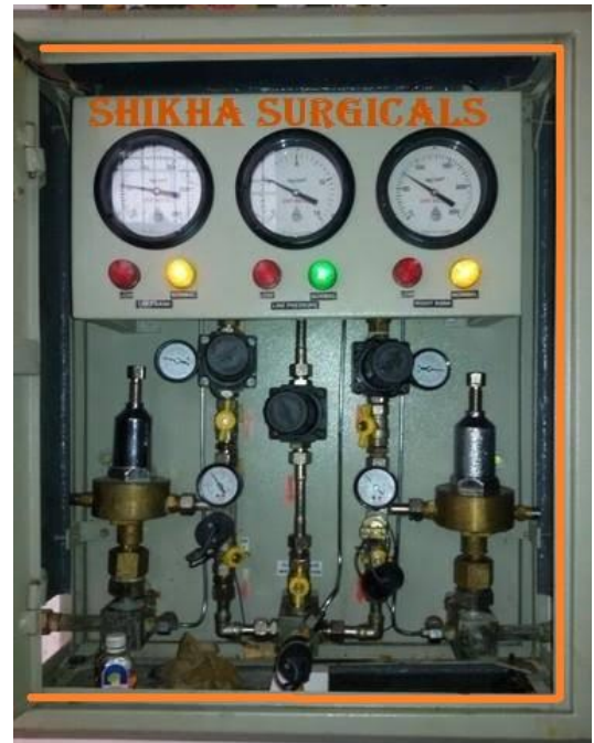
OXYGEN CONTROL PANEL
